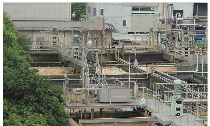
Wastewater treatment facility (Himeji Works)
