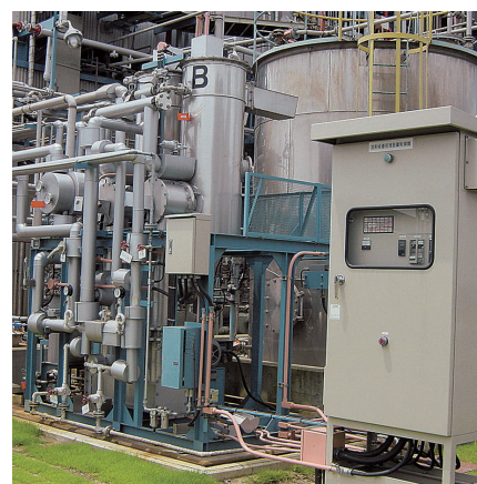
Gas recovery facility (Himeji Works)
