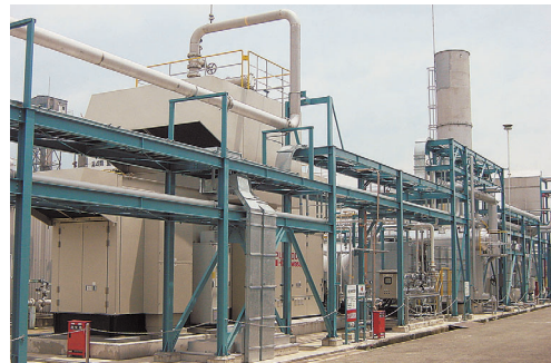
Introduction of a cogeneration system (Himeji Works)
