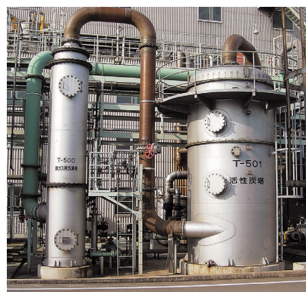
Exhaust gas pollutant removal equipment
