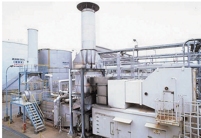
This cogeneration facility also contributes to reducing the amounts of SOx and particulate matter (Befu Works)
