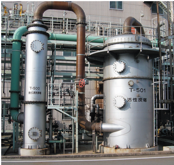
Exhaust gases pollutant removal equipment
