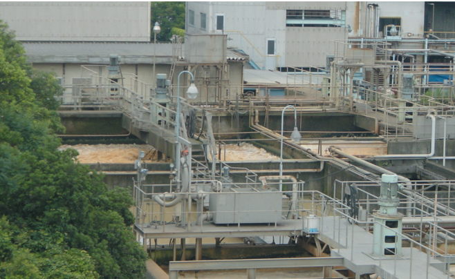
Wastewater treatment facility (Himeji Works)
