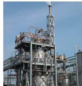
Waste-incinerating volume-reduction plant
