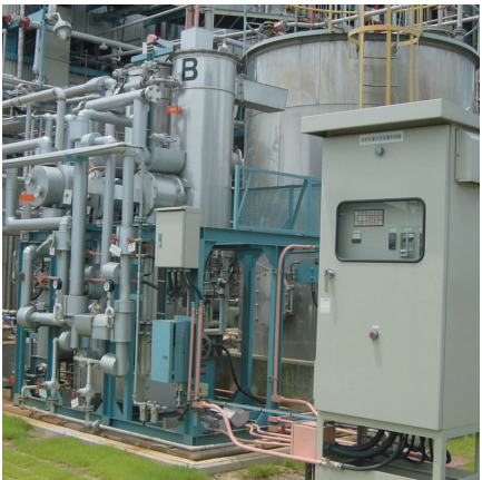
Gases recovery facility (Himeji Works)
